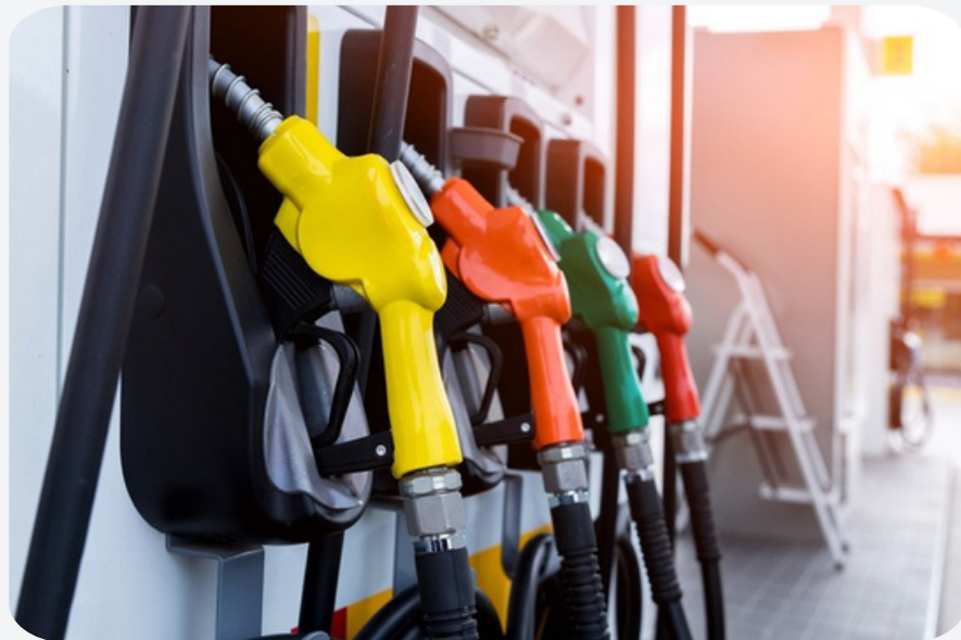
Fuel station- CNG/PNG/LPG
