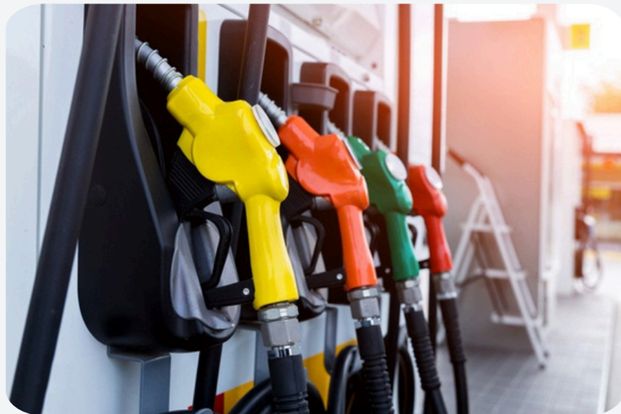
Fuel station- CNG/PNG/LPG
